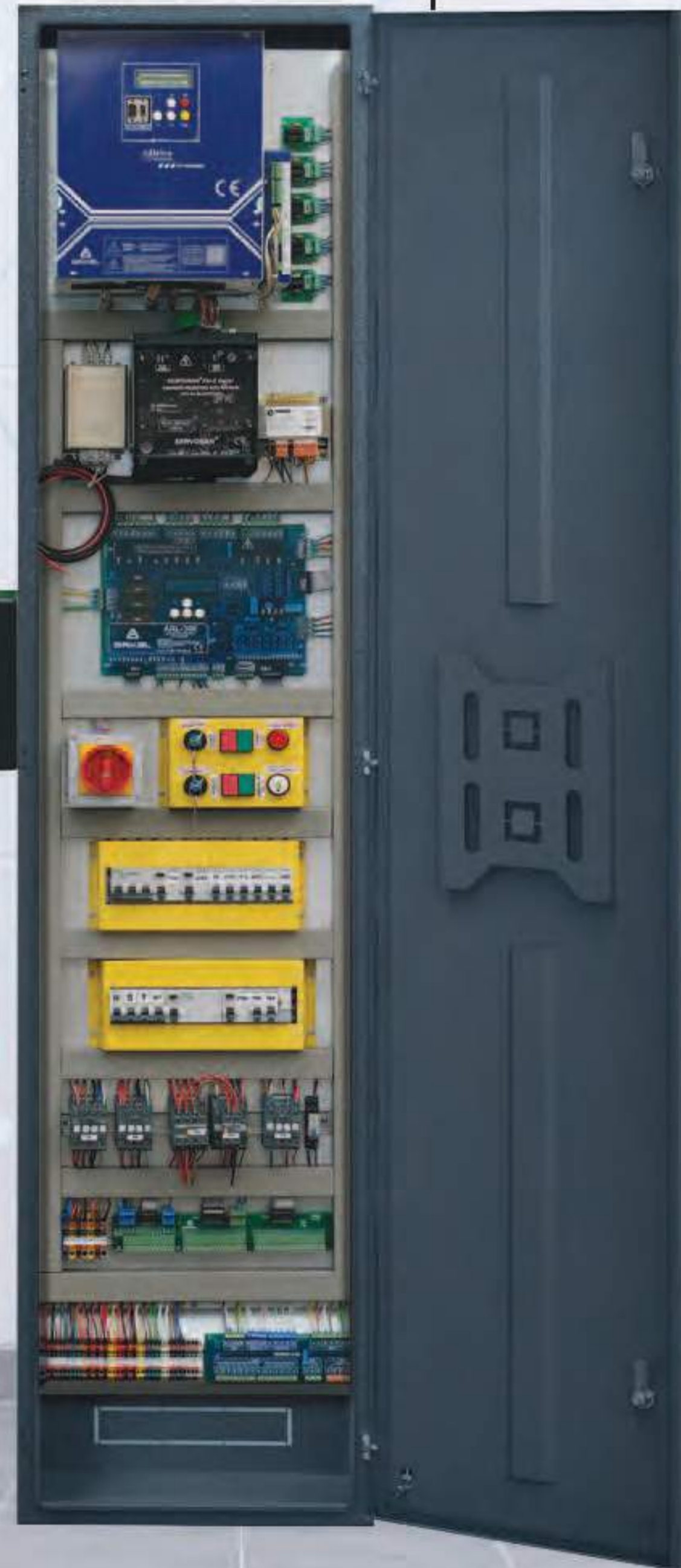
Dişlisiz Pano (MRL) Gearless Control Panel (MRL)
