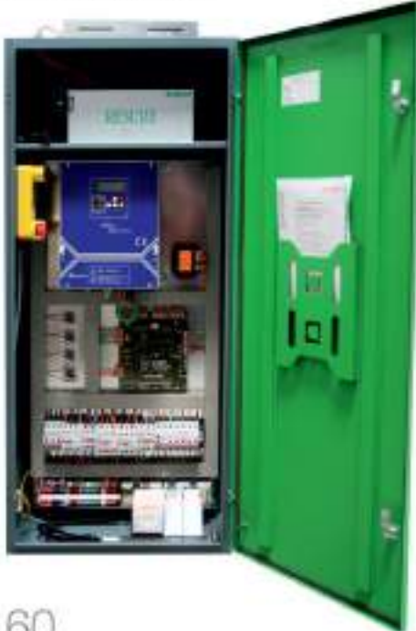
VVVF Kumanda Panosu VVVF Control Panel
